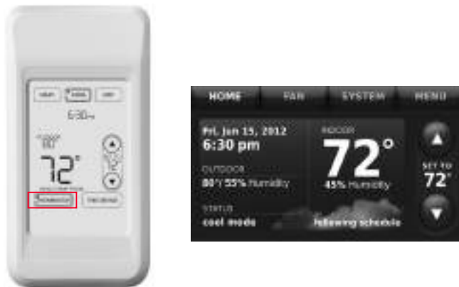
Fig. 312. Reading temperature at the thermostat.
